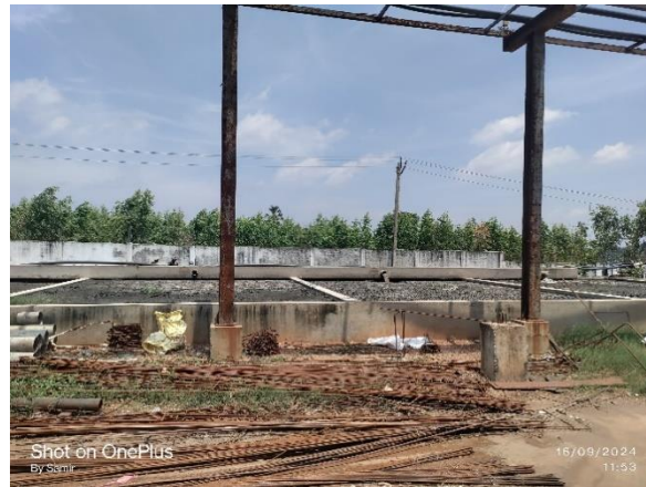
Solid Sludge Treatment
